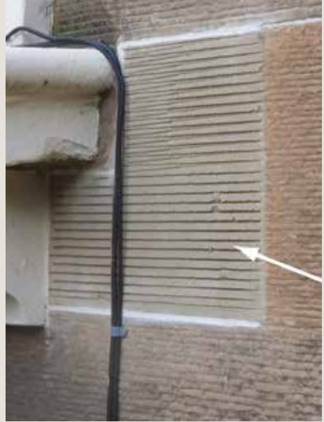
Fig. 10 Surface detailing in the repair (arrowed) does not match the adjacent stone.
