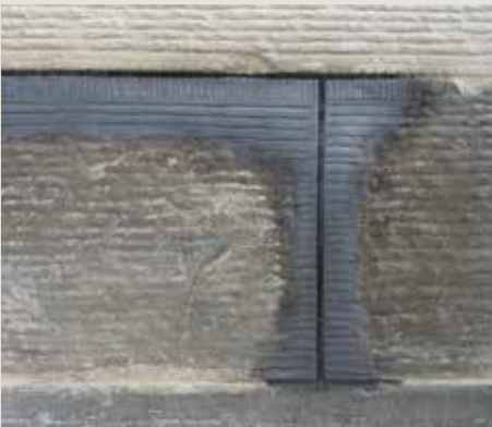
Fig. 7 Restoration mortar colour matched to one area of masonry can be a poor match to another.
