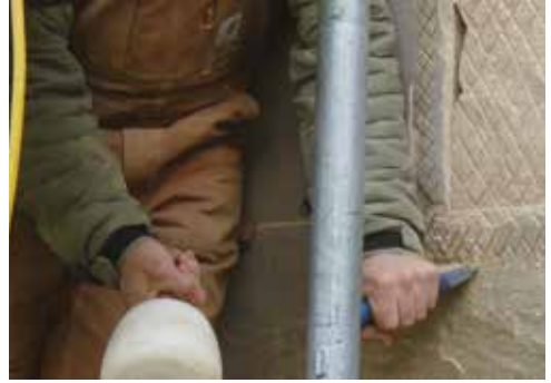
Fig. 6 Surface preparation for application of restoration mortar requires chiselling to a sound surface.
